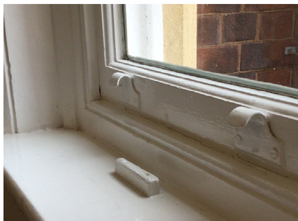
Window frames in the IT corridor still have wartime additions to hold black out screens
